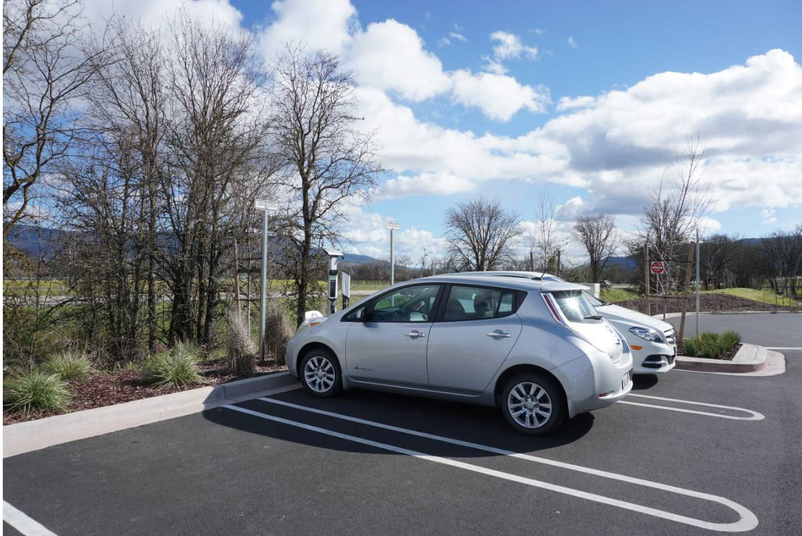
Plate 14 Level 2 charger in the Costco parking lot in Ukiah
