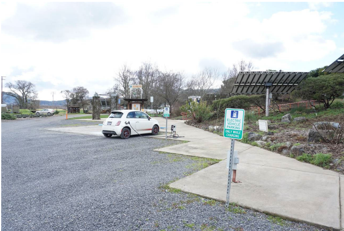
Plate 12 Level 2 charger at EcoTerra Center in Hopland
