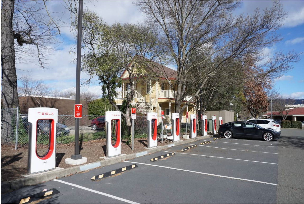
Plate 4 Tesla Superchargers in a City Ukiah parking lot
