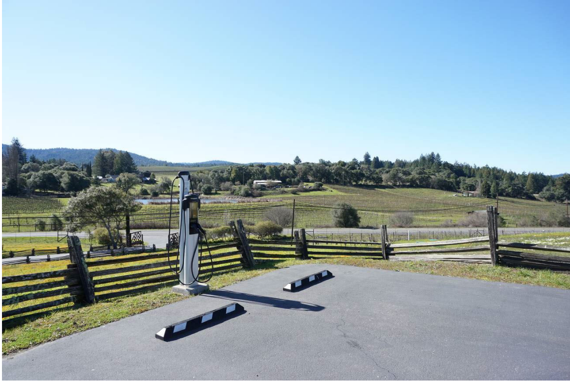
Plate 11 Level 2 charger at Handley Cellars in Philo
