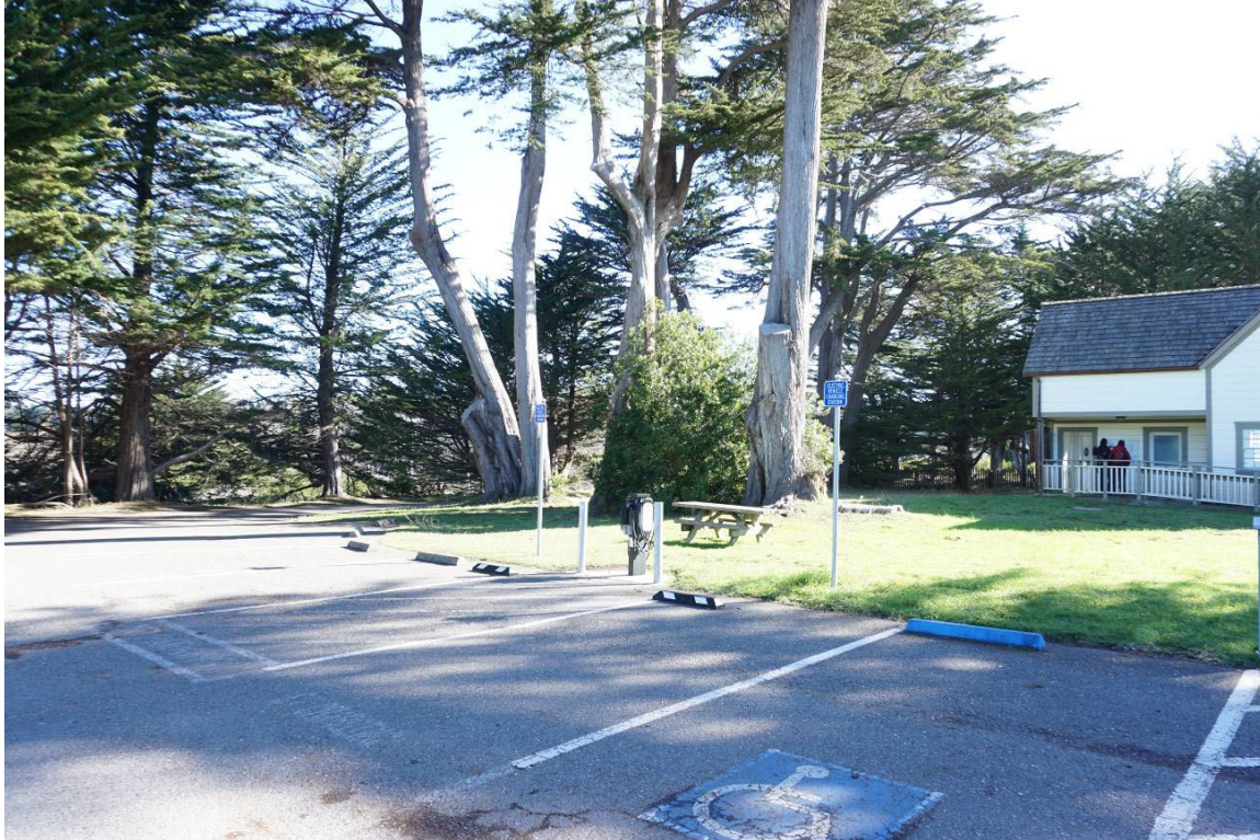
Plate 8 Level 2 charger at the Cabrillo Light Station State Historic Park
