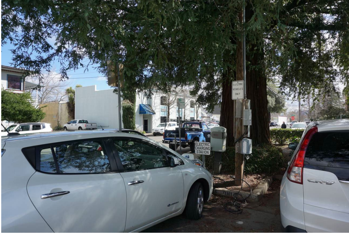
Plate 13 Level 2 charger in City of Ukiah parking lot
