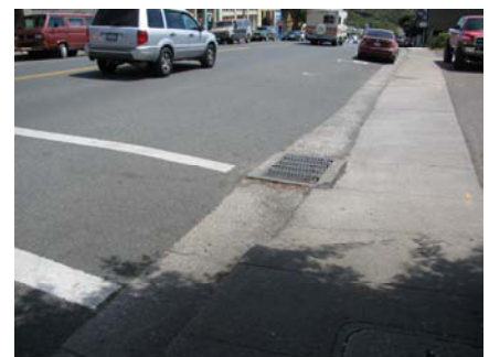
Lack of ADA compliant curb ramp at the mid-block crossing adjacent to the old fire house
