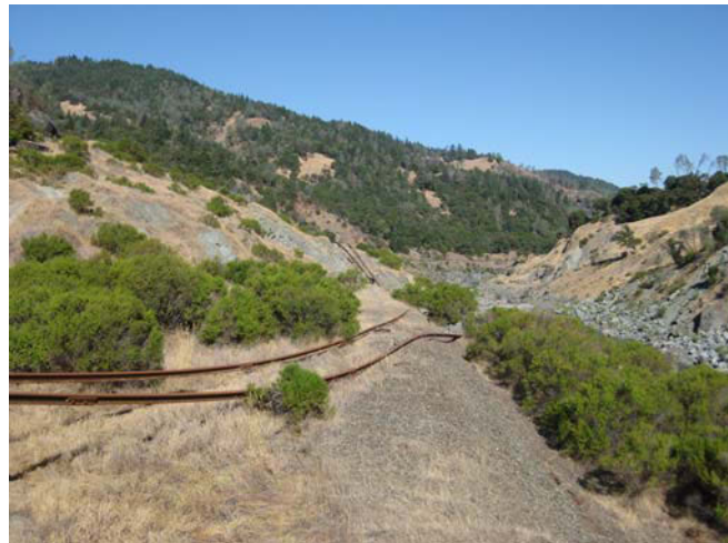
The Eel River Canyon is one of several portions of the NWP rail line that have experienced heavy storm damage
