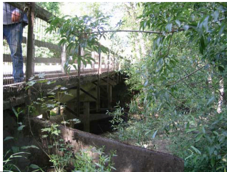
Segment #5 – This is a photo of the underside of the Ten Mile Creek Bridge. The existing walkway is an extension to the current bridge and is not of sufficient design to support equestrians.
